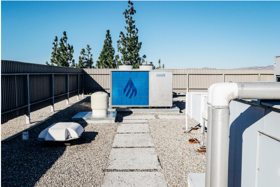
Central heat pump water heater on the roof of Casa Panorama Apartments
